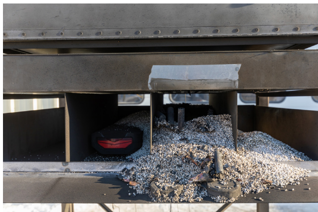
Post test - test sample cubicle and immediately adjacent battery
